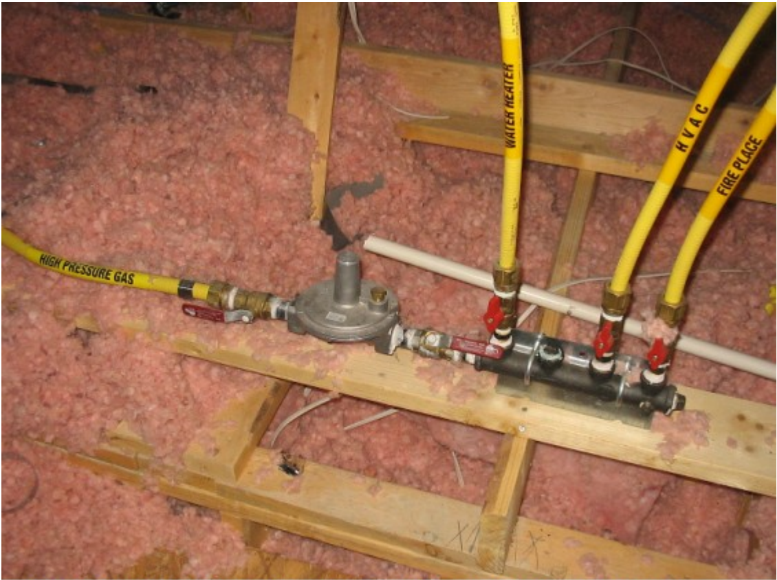
A CSST system with each pipe nicely labeled as to application.
